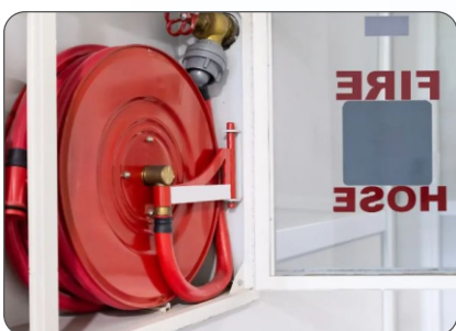
Fire Fighting System
