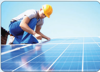
Solar System For Common Area
