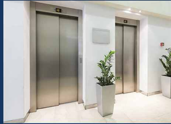
2 LIFTS WITH POWER BACK-UP
